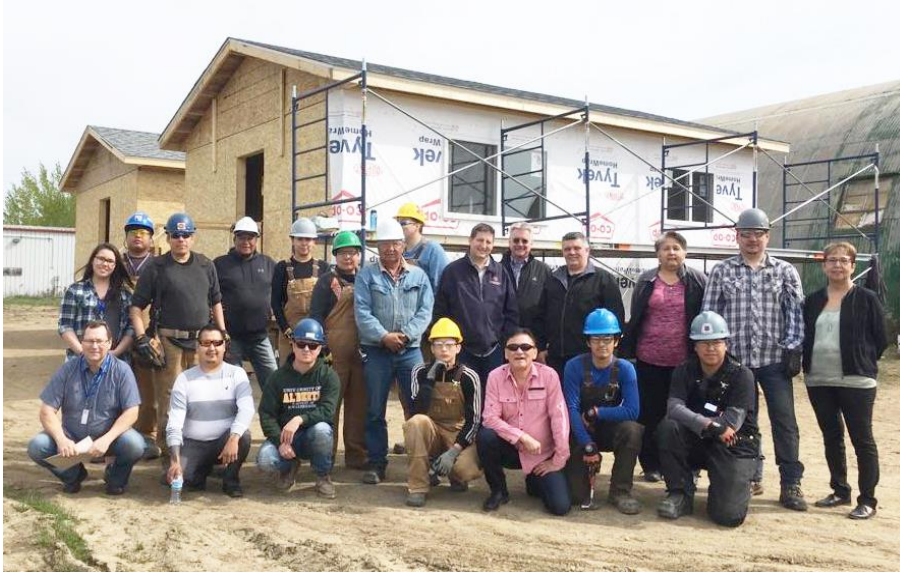
Canadian Natural and the Northeast Alberta Apprenticeship Initiative partnered with the Tribal Chiefs Employment & Training Services Association on the Tiny Homes project. The project brought together employment opportunities and affordable housing developments in areas that lack adequate housing or training required to complete such a feat.
