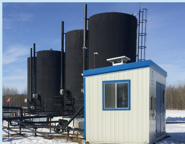
Solution gas conservation compressor unit at our Bonnyville facilities.
